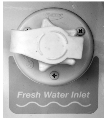
Fresh (City) Water Connection “Fresh Water Inlet” (Located in the water service center)
