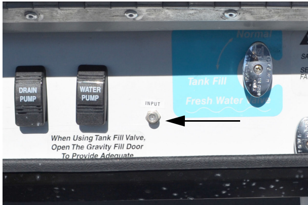
Cable TV Input Connection (Located in Water Service Center)
