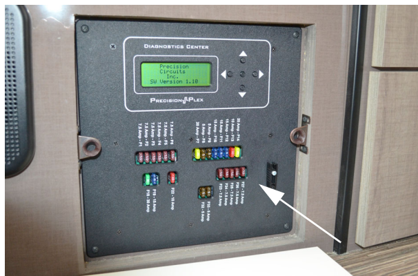
House 12-Volt Fuses -Typical View
