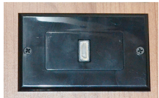
HDMI Connection (Located in cabinet behind TV) -Typical View
