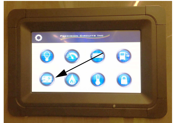
Power Control System
