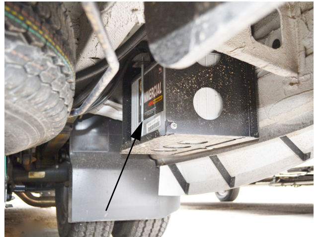
House Battery Access
